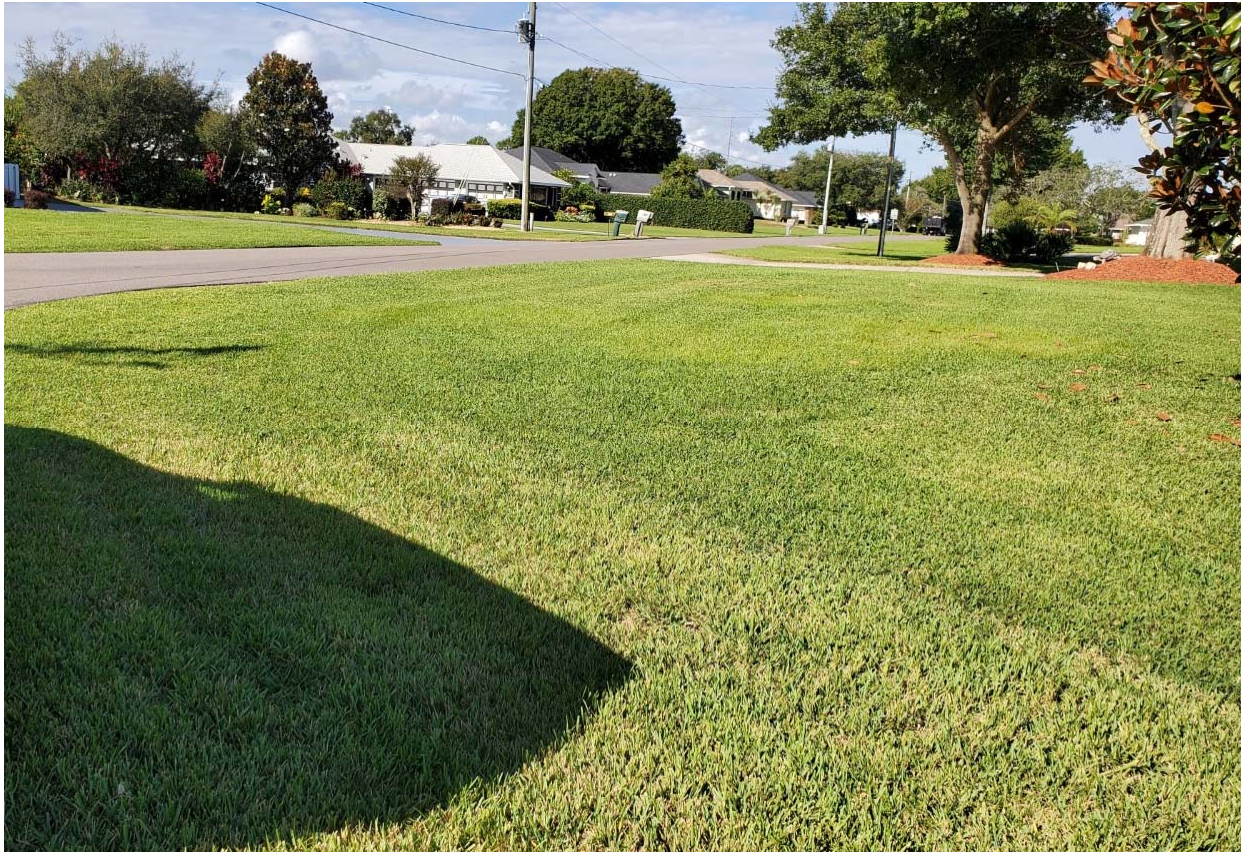
Image of westerly side of the road near the Dog Leg Drive Intersection The ditch is very shallow and the running slope is very little.
